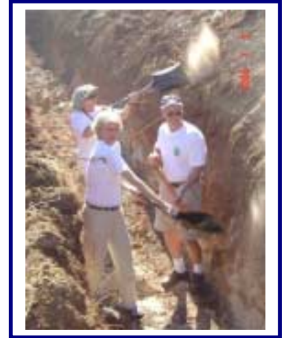
Marie Heintzman, President of the RC of Oakville-West, Gwenn van Schalkwyk, Past President of the RC of Tzaneen, David Angas, Chair of the Rotary Water for Humanity Committee helping dig out a water pipe trench.
